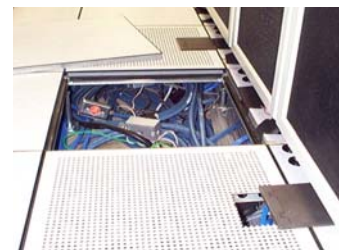
figure 13. Unorganized cables beneath raised floor
