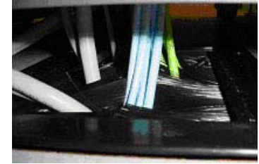
figure 14. Self-sealing cable cutout in raised floor
